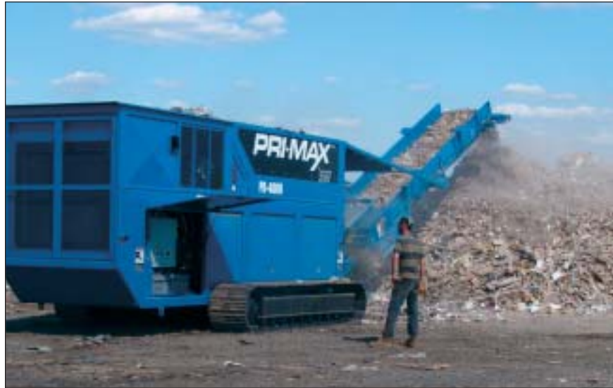
Two passes through the reducer more than doubles the density of the construction and demolition debris stream.
